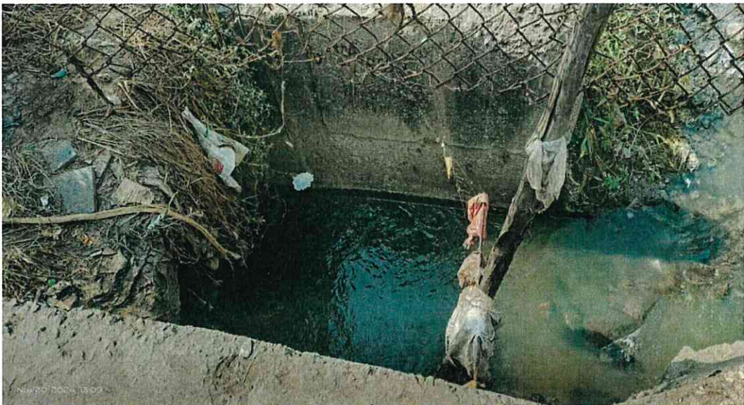
Box drain provided for diverting the sewage from upstream colonies
